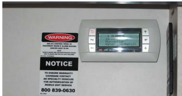
Air Conditioning Trouble Light & Alarm
