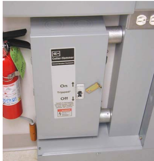
A1 Start/Stop in Equipment Room
