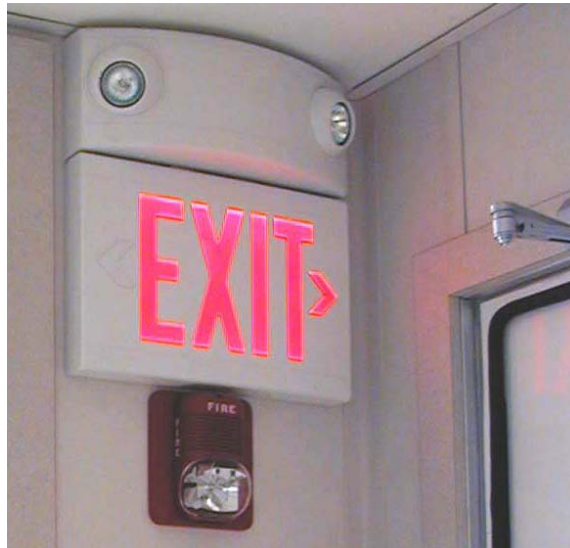
Figure 55: Emergency Dual Beam Lighting
