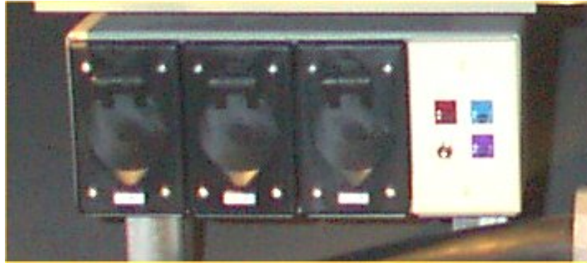
Figure 18: Phone & Data Line Connections
