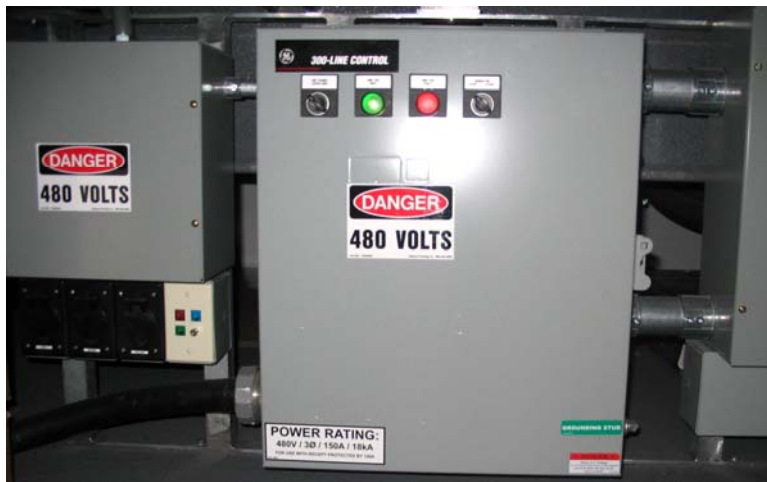
Figure 12: Power Supply Control Panel
