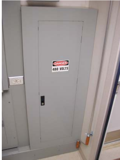
Figure 37: 480V AC Electrical Panel
