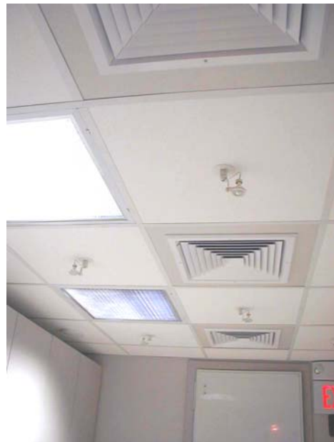
Figure 60: Control Room Lighting
