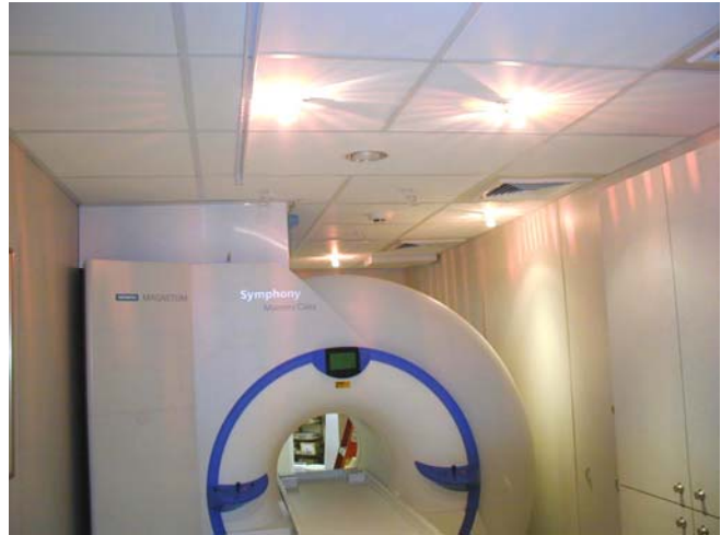
Figure 61: Scan Room Lighting
