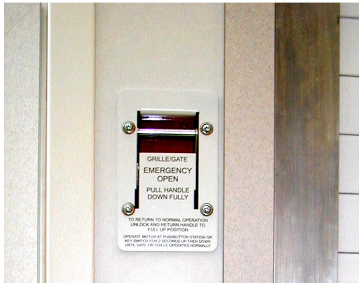
Figure 34: Roll Door Emergency Release
