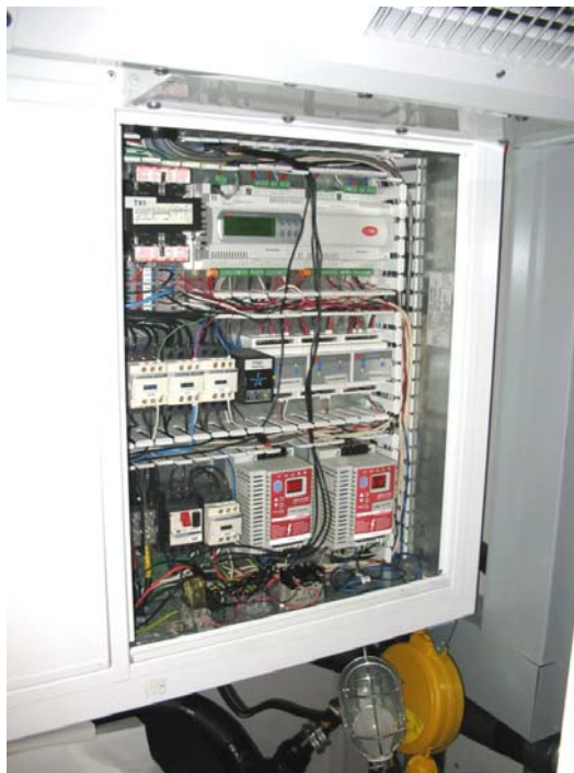
Figure 44: A/C / Chiller Control Panel
