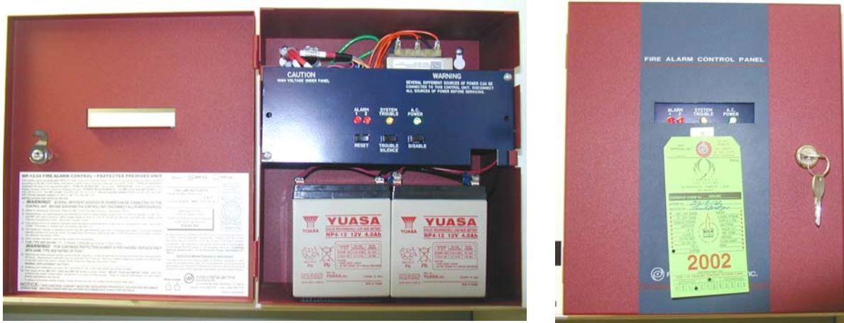
Figure 29: Fire Alarm Control Panel
