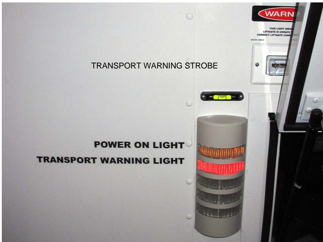
Figure 66: Lift Transport Warning Strobe
