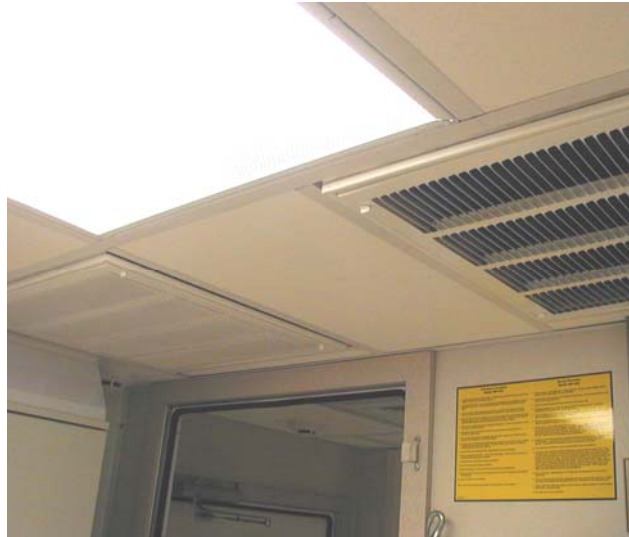
Figure 59: Equipment Room Lighting
