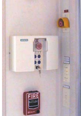
Control Room Lighting and E-Stop and Magnet Quench Controls
