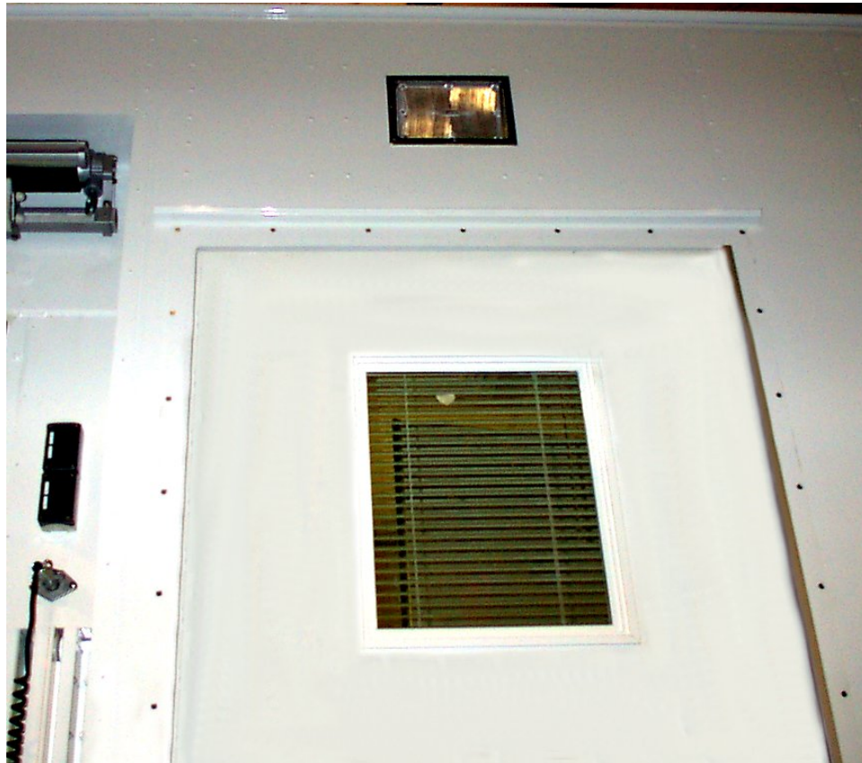
Figure 58: Staff Door Lighting
