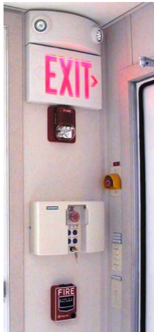
Emergency Off button, Control Room, next to Entry Door
