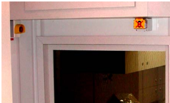
Scan Room E-Stop and Magnet Quench Controls
