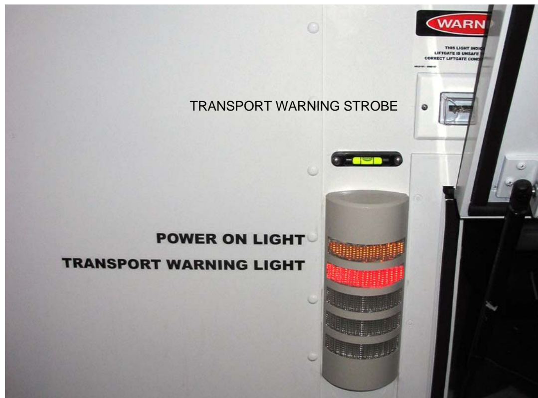
Figure 64: Lift Transport Warning Strobe
