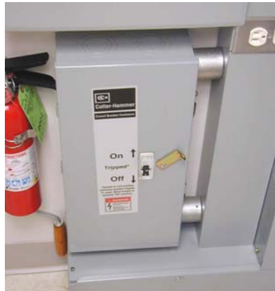
Figure 38: A1 Electrical Panel
