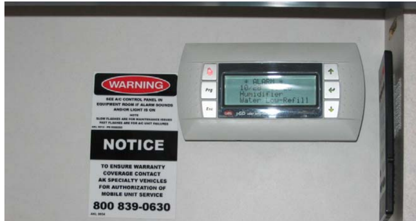
Figure 45: A/C / Chiller Alarm Panel
